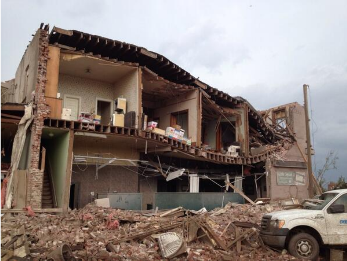
Figure 15: Total collapse of exterior wall along south side of Midwest Bank. Note the clean failure edge, suggesting little if any positive attachment existed between the south wall and the perpendicular east-west walls, or between the roof and the walls.
