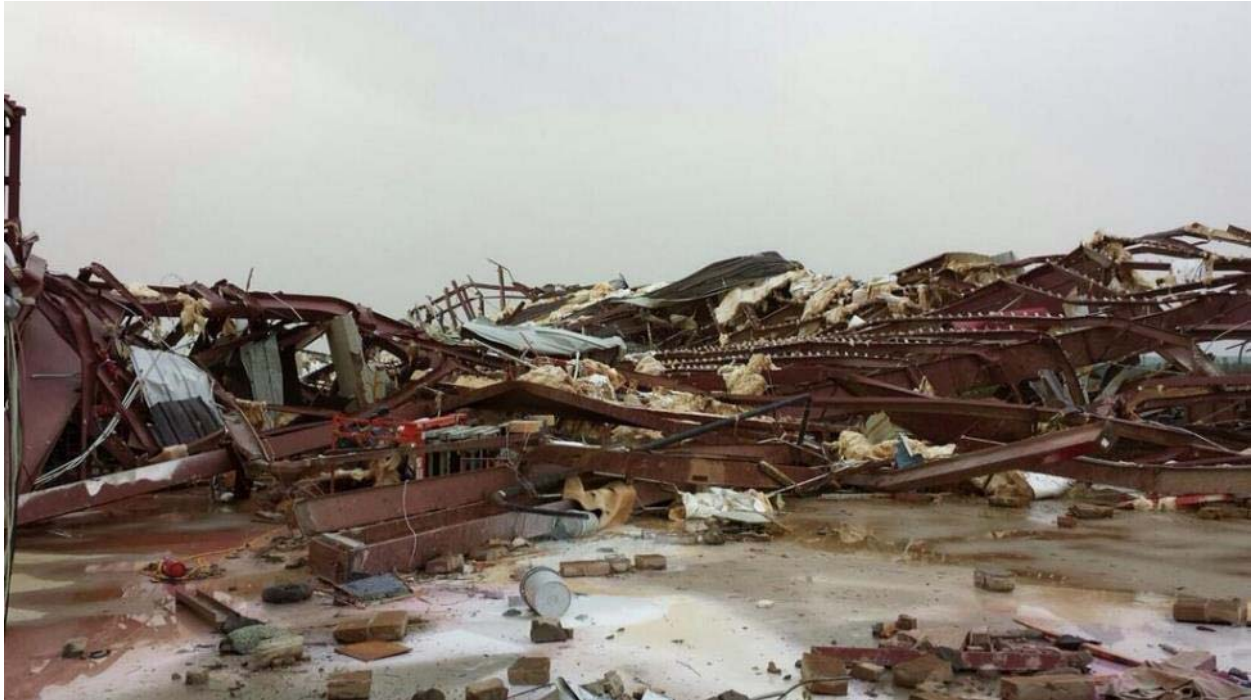
Figure 15. Collapse of structural members at the Intermediate School in Vilonia, AR.
