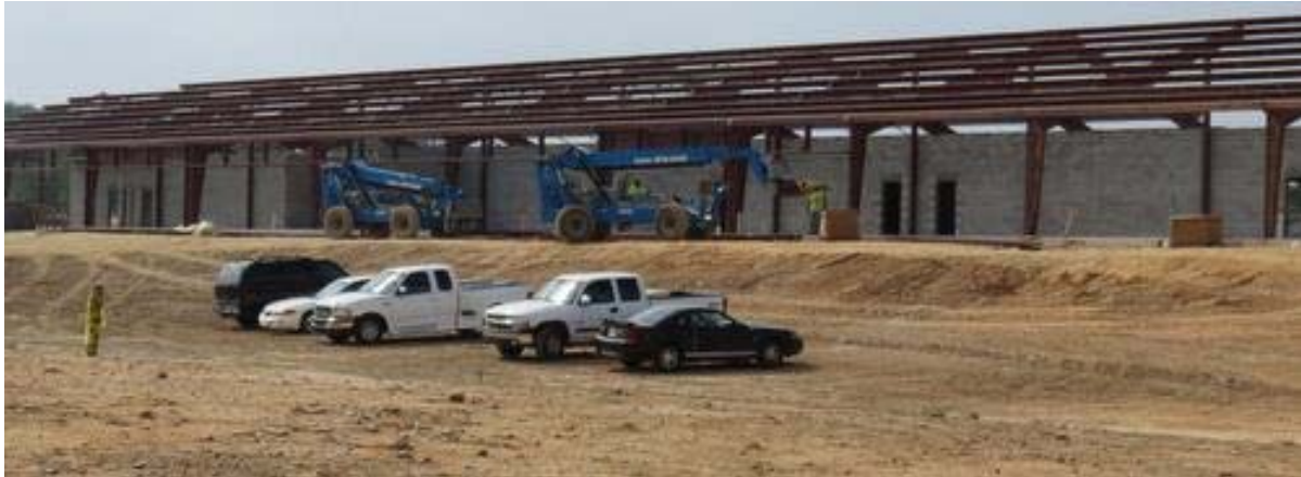
Figure 13. New Intermediate School in Vilonia, AR while under construction. Photo was taken September 29, 2013 by Linda Hicks.
