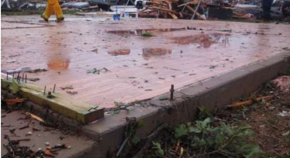
Figure 10: Complete destruction of home with anchor bolts just south of Hwy 377 & N. of Acton Highway in Granbury, TX (Image Courtesy of http://www.srh.noaa.gov/fwd/?n=tornadoes051513 )
