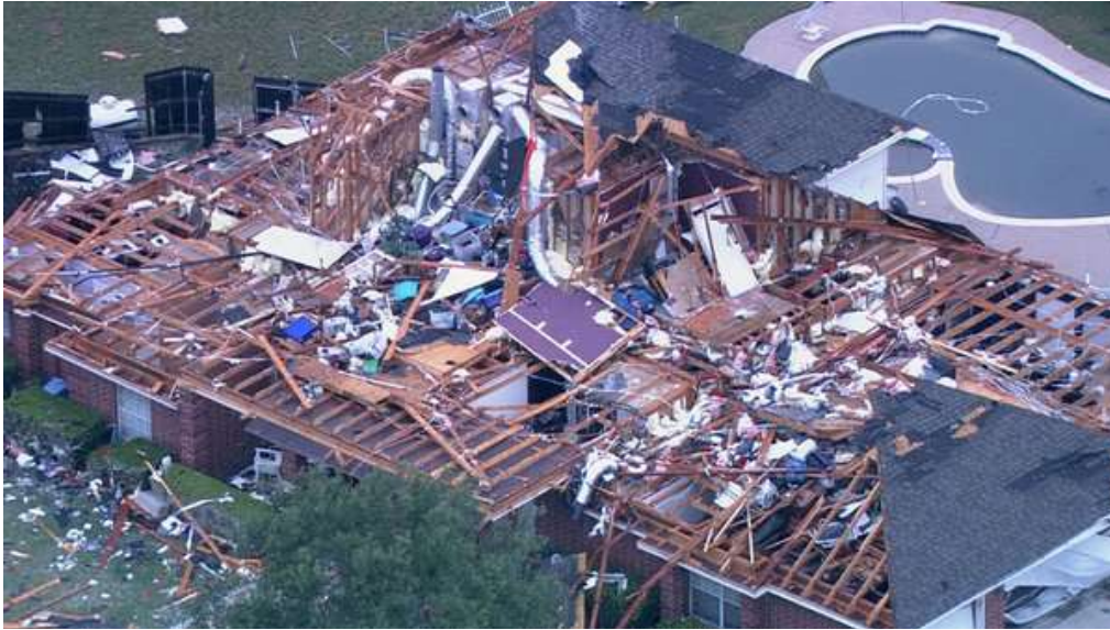
Figure 12: Damage in Cleburne, TX (Credit: WFAA)
